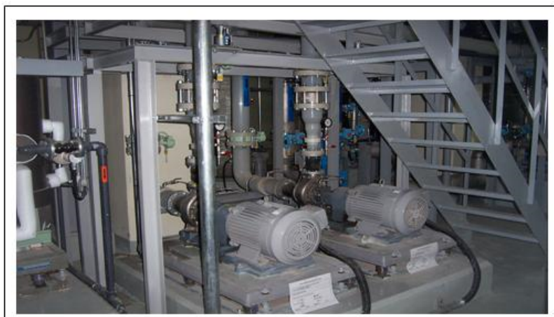
HOT-DI system PUMP
